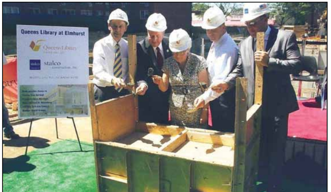
Pictured above putting the finishing touched on the foundation, of the Queens Library at Elmhurst, that will support a wonderful state-of-the art library that will include a Memory Wall and original building bricks to acknowledge the past as well as building for the future is, FAIA Commissioner of the New York City Department of Design and Construction David Burney, Queens Borough President Helen Marshall, Council Member Daniel Dromm, Library President and CEO Tom Galante and Architects and Stalco Construction, Inc. representative Marpillero Pollak. Photo by Bob Grant
